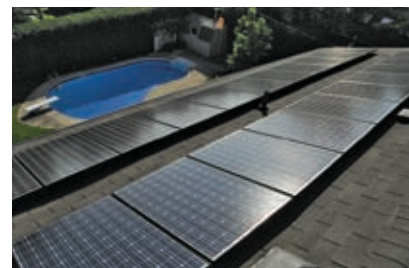
Figure 6: Solar PV Roof-Mounted Array Source: Enviro-Energy Technologies Inc. 8
