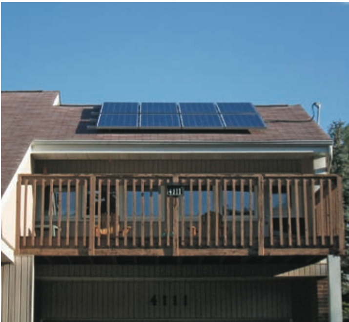
Figure 10: Roof-Mounted Solar PV Array Source: Enviro-Energy Technologies Inc.
