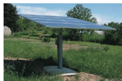
Figure 7: Pole-Mount Solar PV Array Source: Enviro-Energy Technologies Inc.
