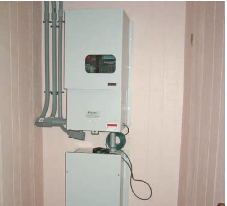
Figure 11: Grid-Interactive Inverter & Battery Bank Source: Enviro-Energy Technologies Inc.
